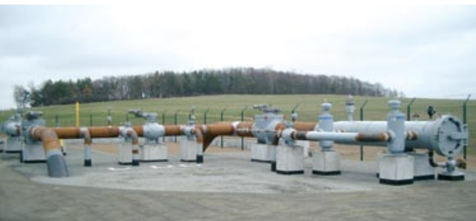
Neue Station Lüptitz
