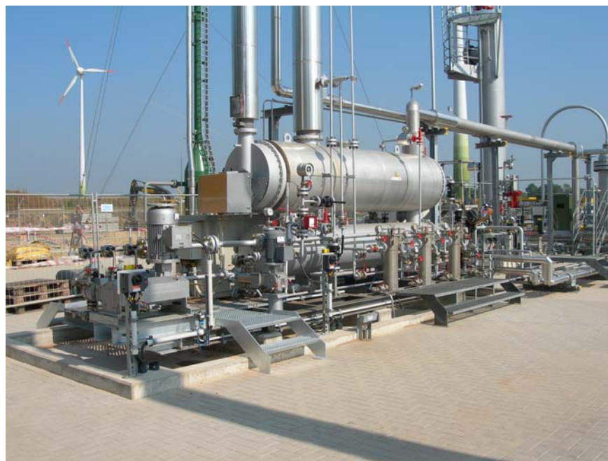
Glycol regeneration unit
