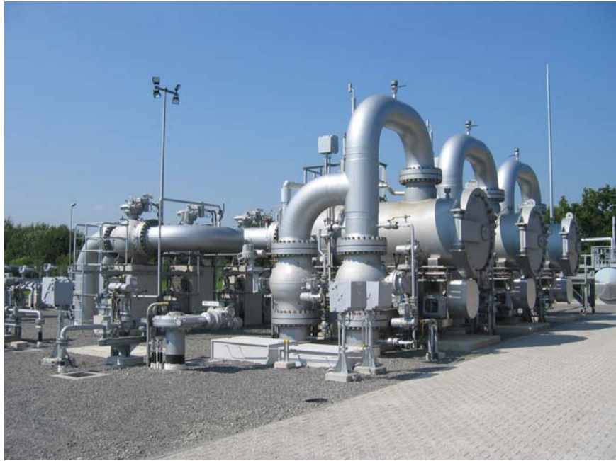
Filter system: 3 separators, pipe diameter 28"
