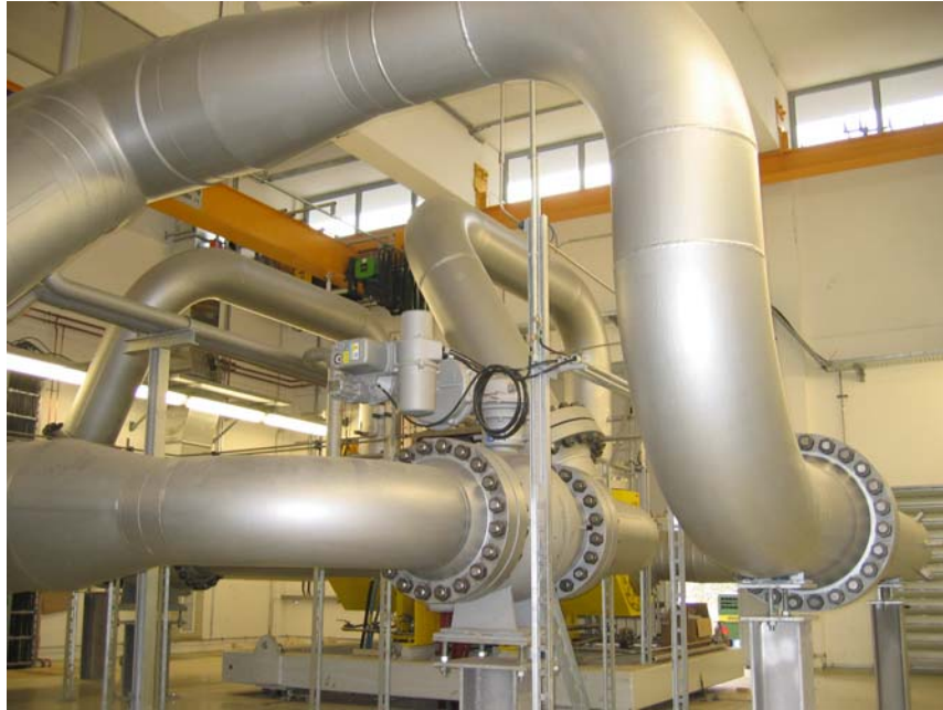
Piping in compressor building, nominal diameters 18", 20" and 28"
