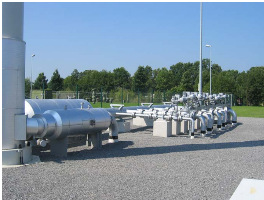
Vent system with vent stack and silencers
