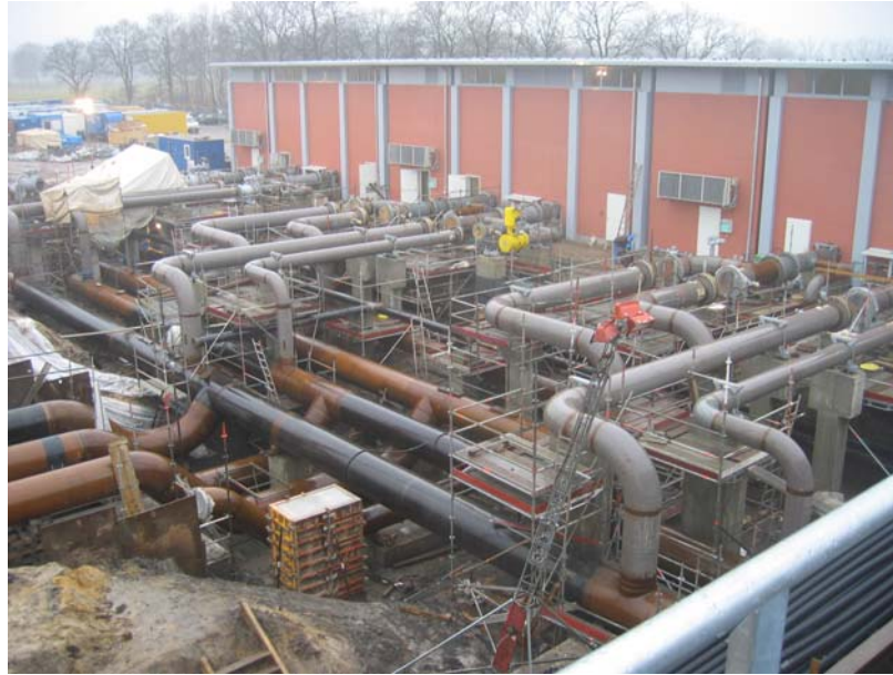
Compressor inlet and outlet manifold in front of the compressor building (ND 40" and 42")
