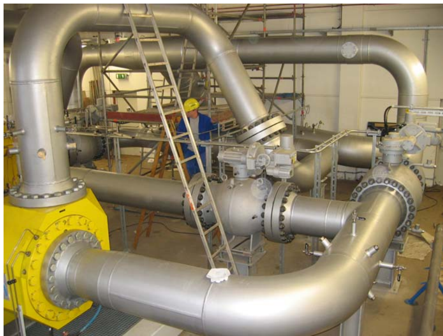
Piping in compressor building, nominal diameters 18", 20" and 28"
